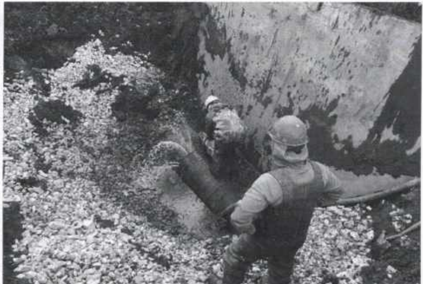
Existing 30-inch main
